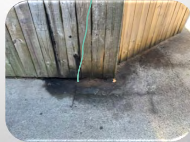
Evidence of discharge from compressor
